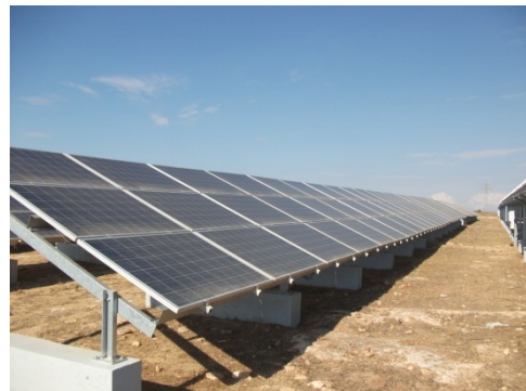
Figure 4. View of solar plant in Serhatkoy, Cyprus
