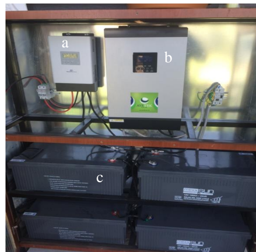
Figure 7. (a) Charge regulator, (b) Inverter, (c) Batteries
