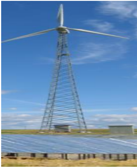
Figure 6. Renewable power plant created in Silifke-Turkey
