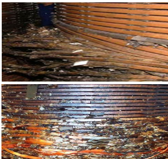
Figure 1. The winding failures detected in the breakdowns of the transformer centers in the Erdemli and Silifke districts of Mersin.
