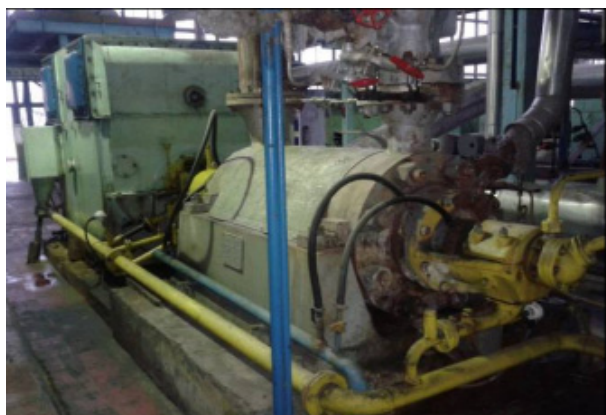
Figure 2. The motor-pump unit [1]
